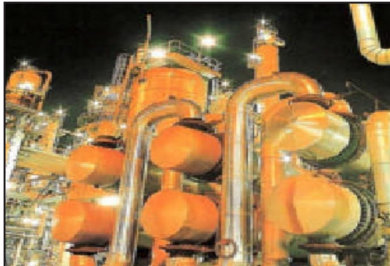
Refinery heat exchangers
